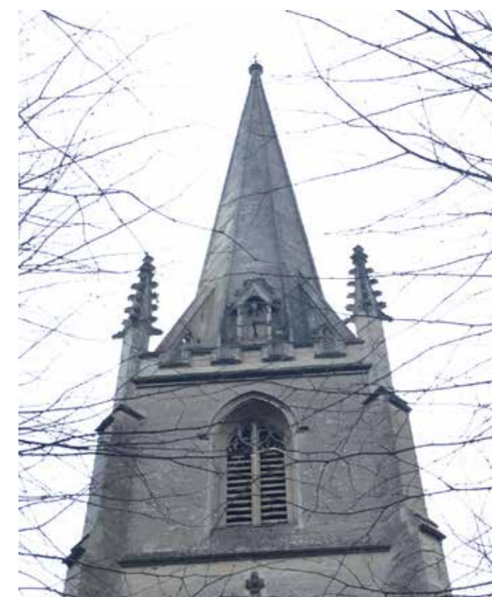
A grant of £2,500 has been made towards the cost of repairing Christ Church clock
