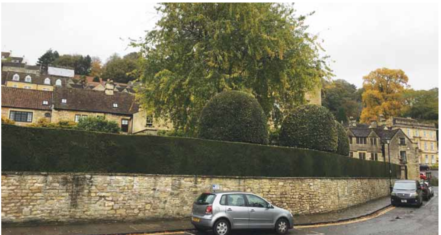
The wall in question – and no trace of the repair, 60 years on
